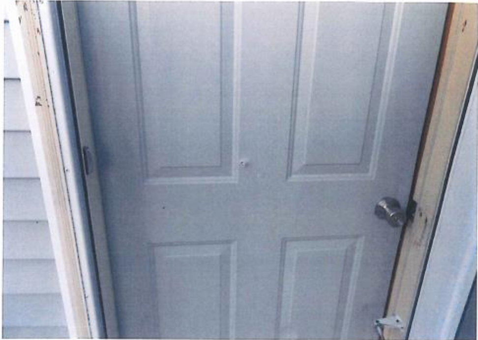
EXHIBIT 5: Third Photograph of Lommy Green’s Door
